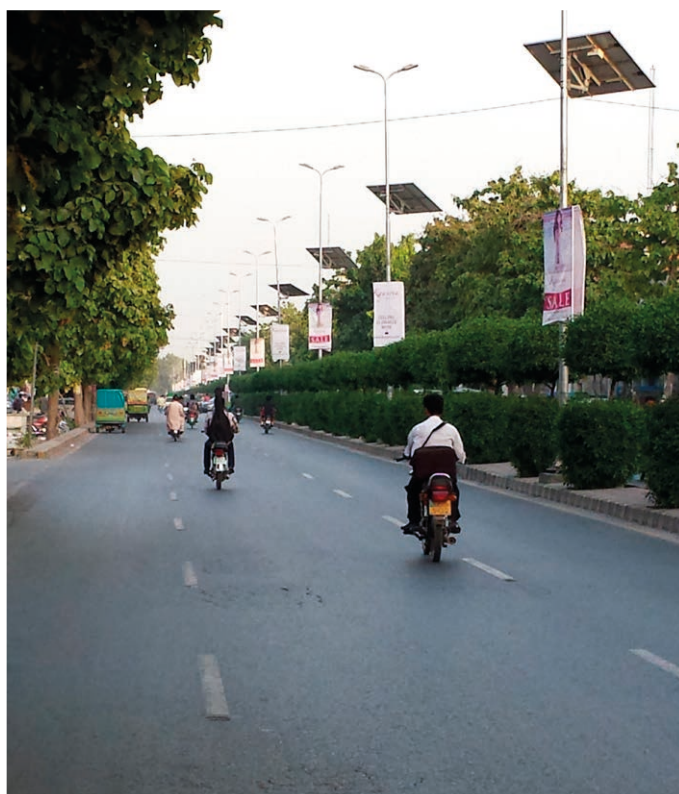
Solar street lights installed on a busy road in Lahore, Pakistan.
