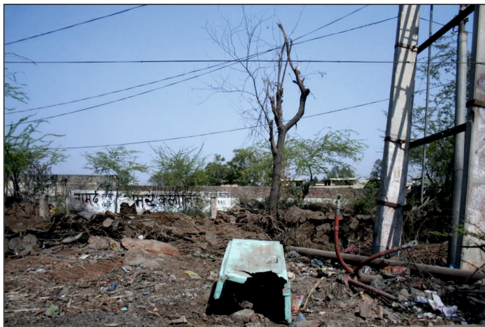
The state of Electricity Infrastructure
