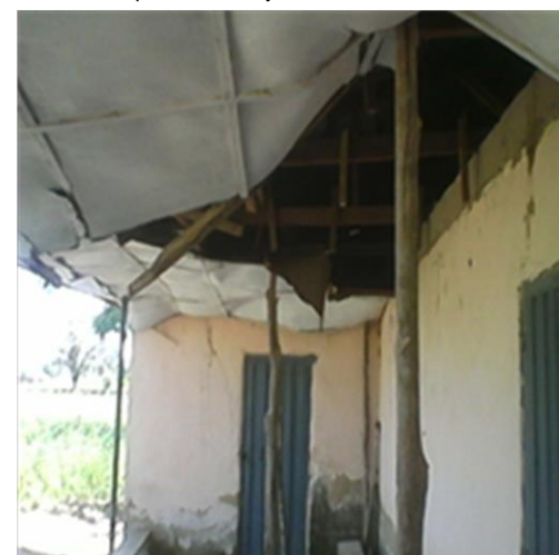
Below: Dilapidated facility at Iri Gida, Kaduna State
