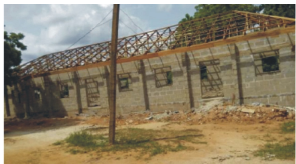
Project Description NBARR16745523, Okongwu Assembly Hall in Okongwu Memorial Grammar School Nnewi, Nnewi North is in progress even to the roofing level. Project Amount is N30M.
