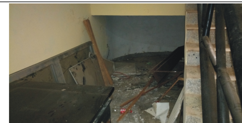
Evidence of abandoned work at FERMA state office
