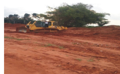
Road project under construction and the point where there was clash between Nkpor and Umuoji indigenes
