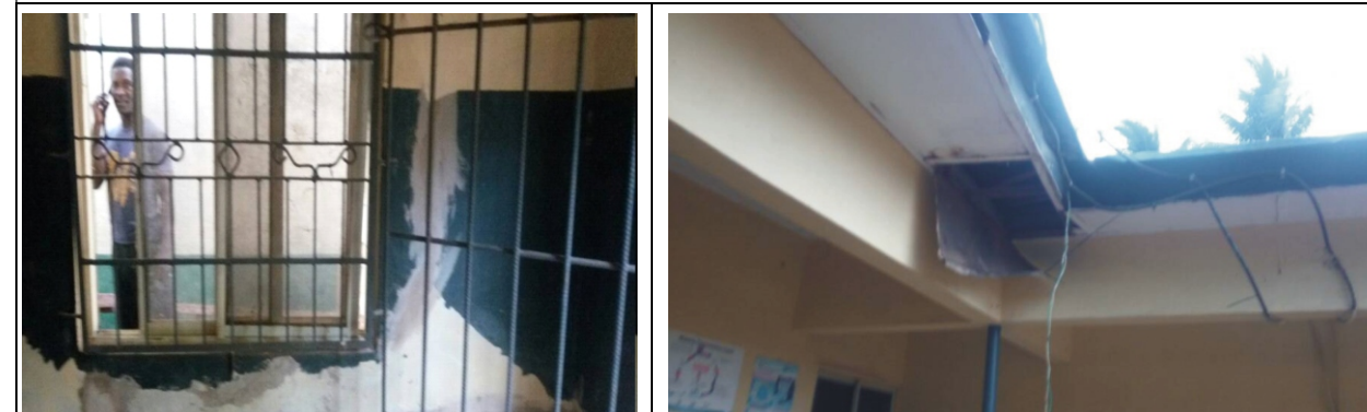
Collapsing and worn out segment of Ukpo Primary Health Care Centre.
