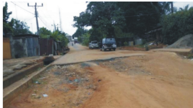
Construction Ikemba Drive, Nothing has been done concerning the project that leading to the permanent site of Nnamdi Azikiwe Teaching Hospital and Project Amount is N400,000.00 (Abandoned)
