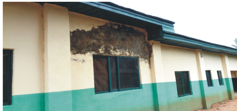
Completed building with substandard painting
