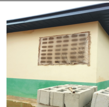
Hollow block window with substandard netting
