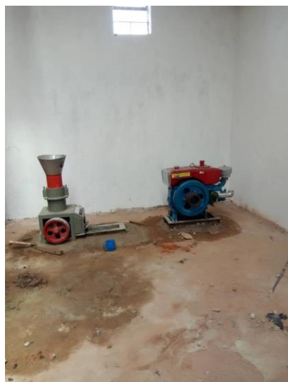
Picture 1: Pellet machine after installation.
